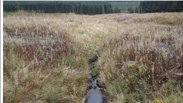
View downstream (SE) showing watercourse valley, rocky channel and existing culvert pipe
